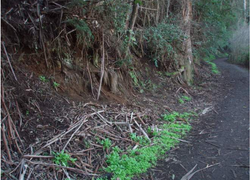
Plate 5. Track cutting on Pipeline Track, Romilly Street/Stoney Steps Road site, where several dead specimens have been found in loose soil.
